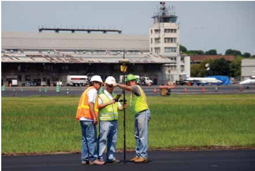
Surveyor Jamie Lovaglio and Super John Carollo are checking finished grades with Topcon dealer Jim Cleary.
